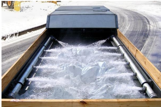
Fig. 15. Hot water spraying system in the melting tank [2]
