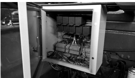
Figure 5: Detail view of the electric control subsystem mounted on the vehicle
